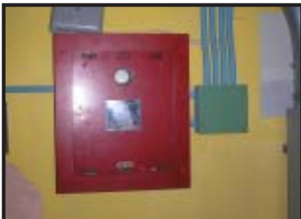
50 Year Old Fire Alarm Panel to be replaced
